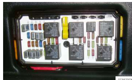
Illustration 217: Electrical box components
